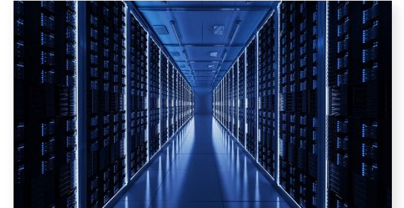
SMART DATA CENTER
